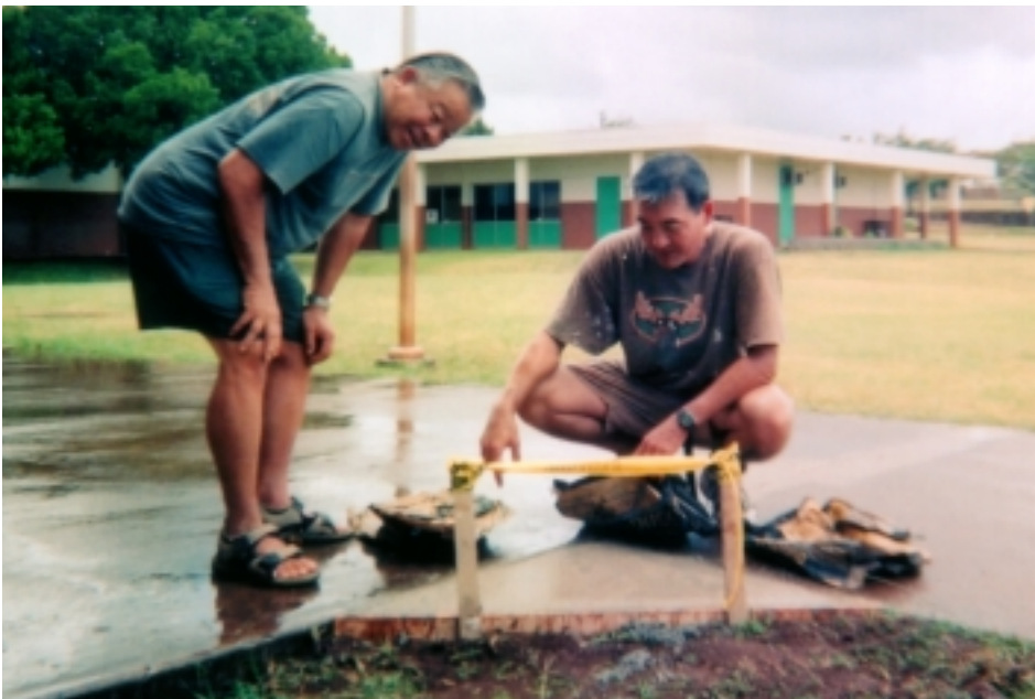
Willie Wong and Eddie Miwa remove cement bags protecting the wet cement from the rain.
